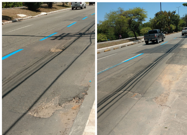
Fig. 32 Sections with poor quality asphalt
